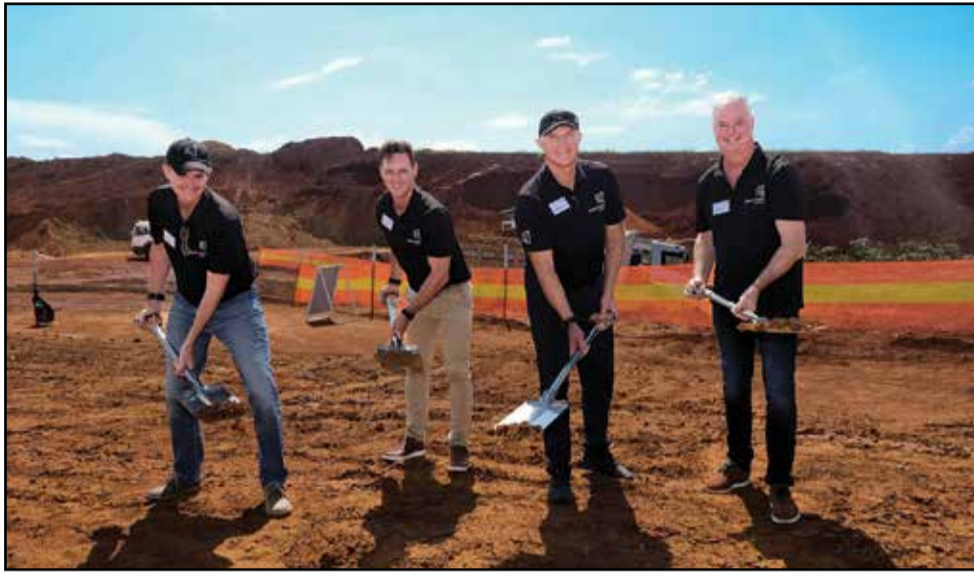
A sod turning ceremony marked the start of development at Growthpoint Properties' Tecoma Park, from left: Jason Reeves, head asset management: Logistics and Industrial Portfolio of Growthpoint Properties, Kobus Blom, KwaZulu-Natal regional development manager of Growthpoint Properties, Estienne de Klerk, SA CEO of Growthpoint Properties and Greg Worst, KwaZulu-Natal regional head of Growthpoint Properties
